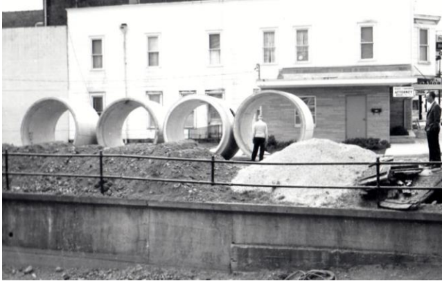
Rev. L. G. Fritz looking at the culverts that will be used to flume the canal.
