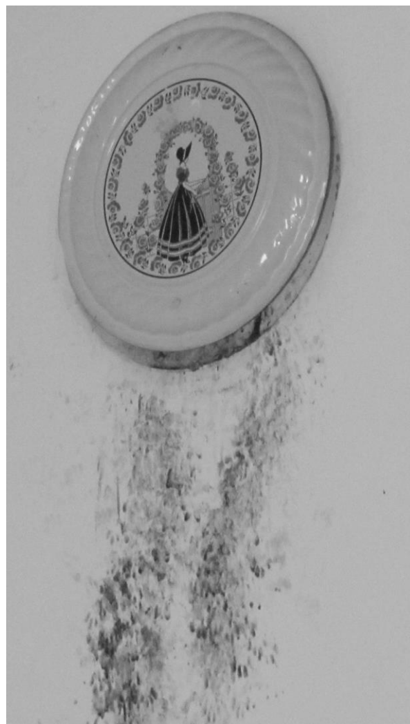
The squirrels' point of entry was marked by tiny footprints on the wall below the stove pipe flue cover.
