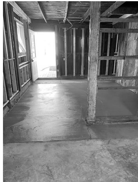
The building has been rewired, the walls ready for insulation, and the floor prepared to accept a covering.
